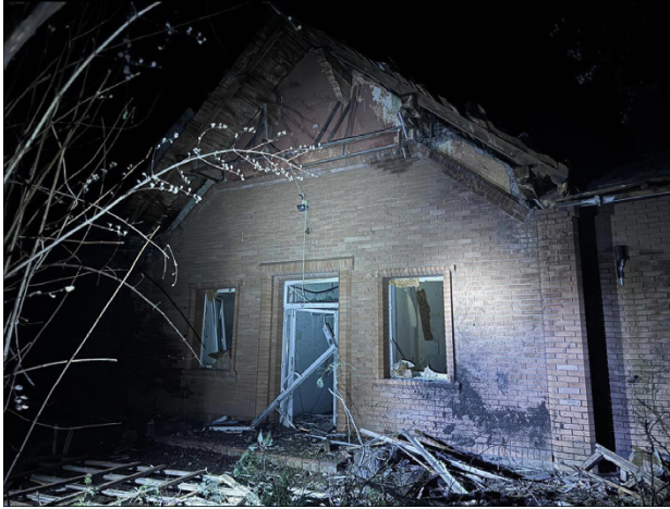
■ Damaged premises of the Ukrainian Red Cross Society. Photo: Facebook
